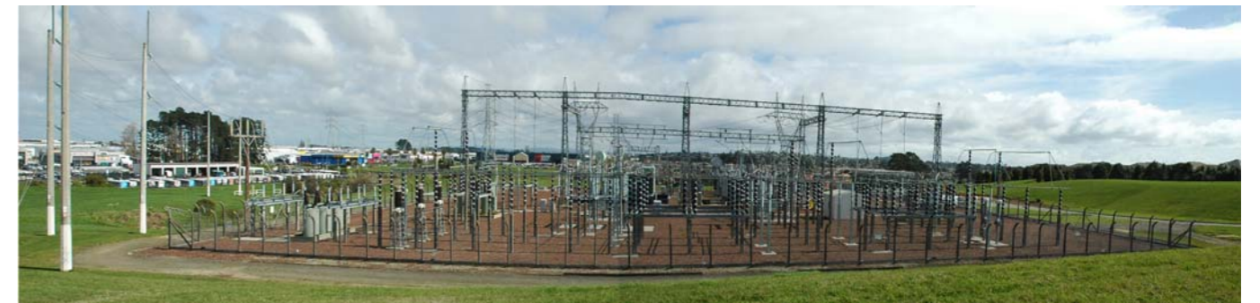
Air Insulated Switchgear at the existing Pakuranga substation
