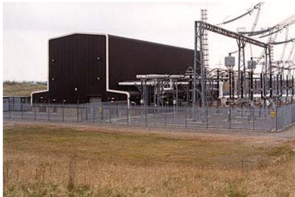
A Gas Insulated Switchgear substation
